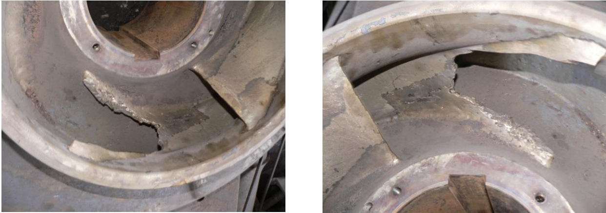
Figure 13. Cavitation erosion on the impeller blades of the storage pump
